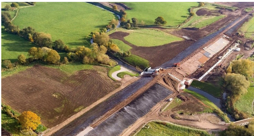
Figure 9: Working in partnership with Lancashire and Chorley Councils “Croston Dam” protects 400 homes and businesses from flooding.
